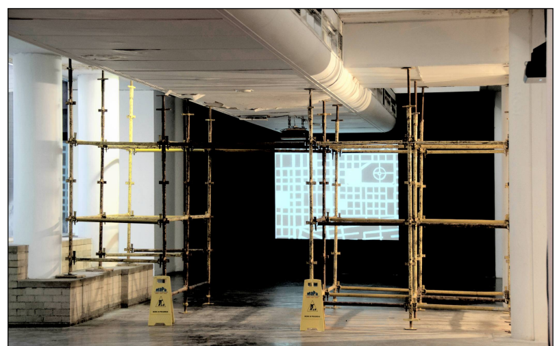
Scaffolding (all three pics above) around a leaking roof is the centre of Hobbs's Jagsnag project.
